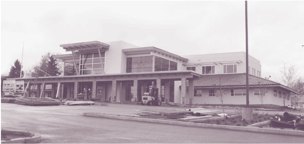
Construction of the new combined dental and medical facility (left) in Yakima is almost complete.
